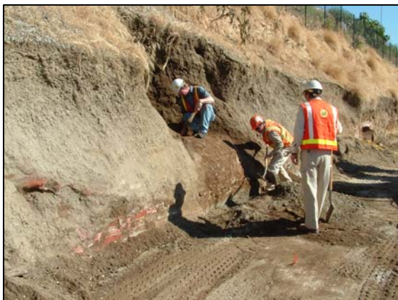
Day Two: Segment of Zanja uncovered by MTA laborers under supervision of Cogstone archaeologist. The zanja is constructed of a double course of brick with mortar and is about 3.5' in diameter.
